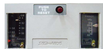
Example of High/Low pressure safety
